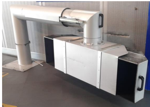
6 Fume extraction system
